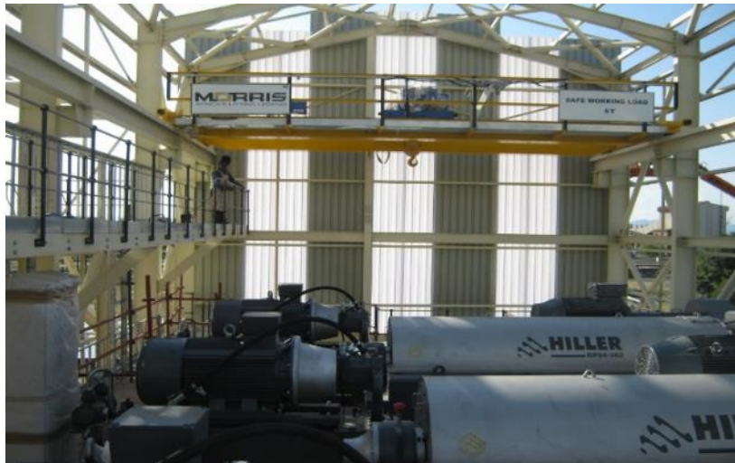
Dewatering plant at Zondereinde
