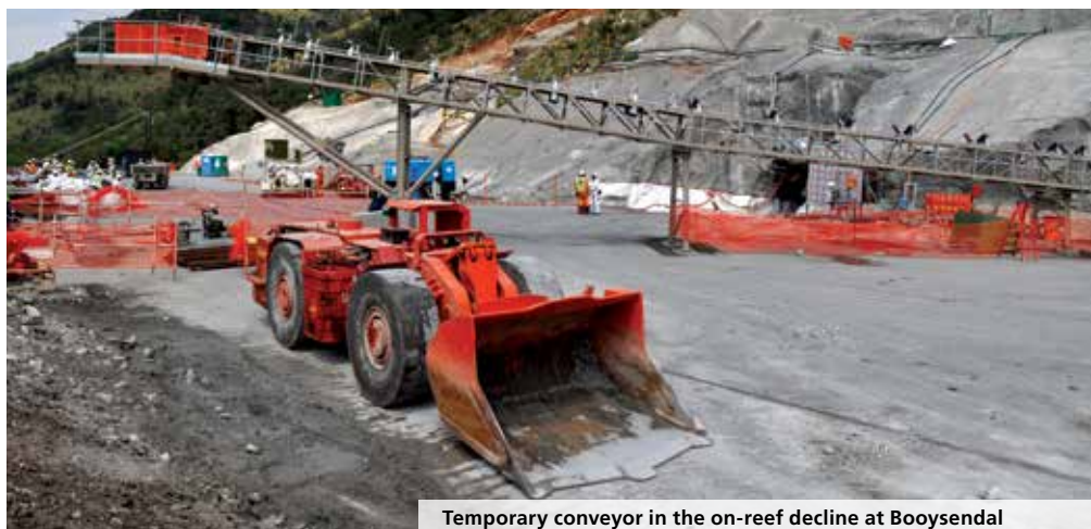
Temporary conveyor in the on-reef decline at Booyssendal
